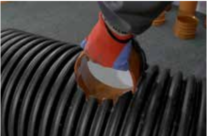
7. Inserting body of sag through pre-prepared opening and setting int in the appropriate position
